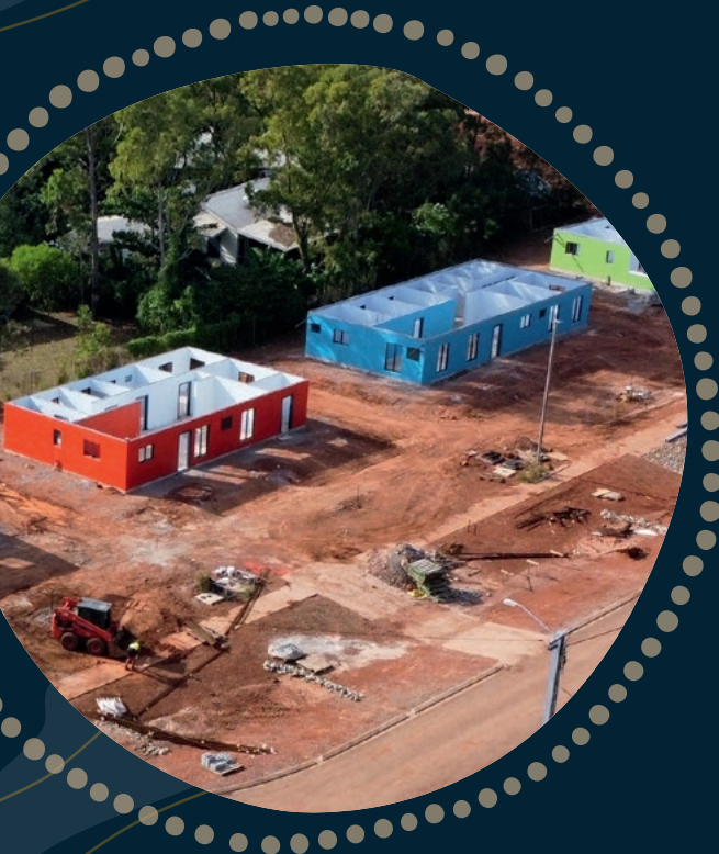
Homes under construction in Yirrkala, Northern Territory. Photo courtesy of the Northern Territory Government.
